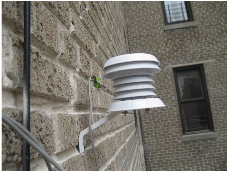
Figure 5 – Exterior Air Temperature Sensor Photo
