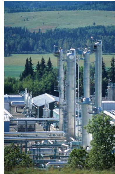
Gas power plant.
