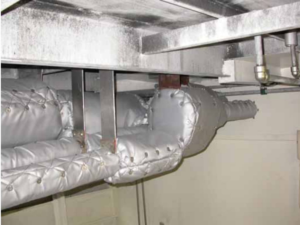
Figure 2.18. MV PORT IMPERIAL MANHATTAN Exhaust System in Lazarette.
