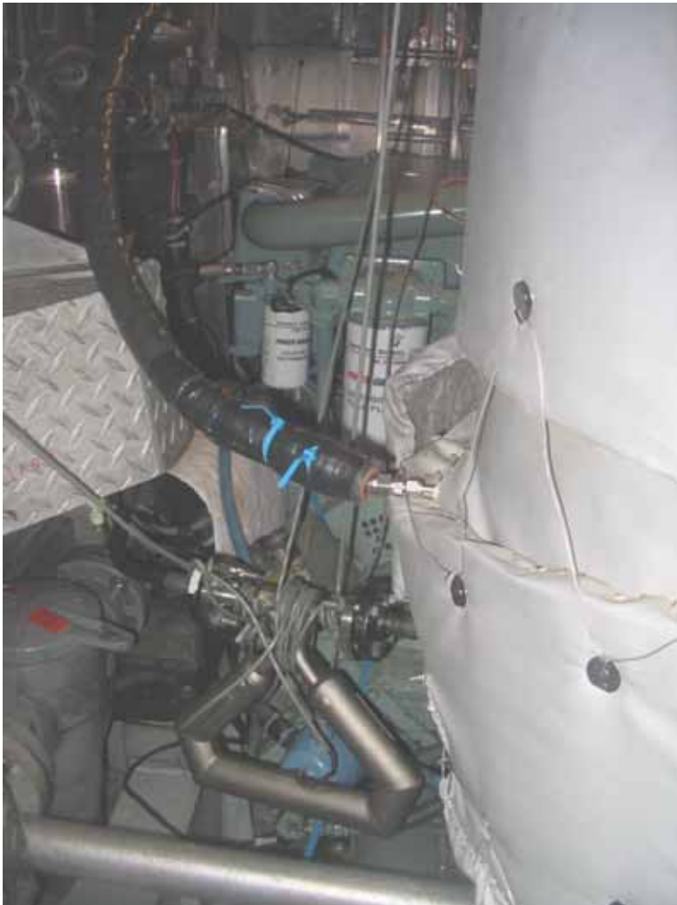
Figure 5.3. MV JOHN KEITH Engine Room Looking Forward.
