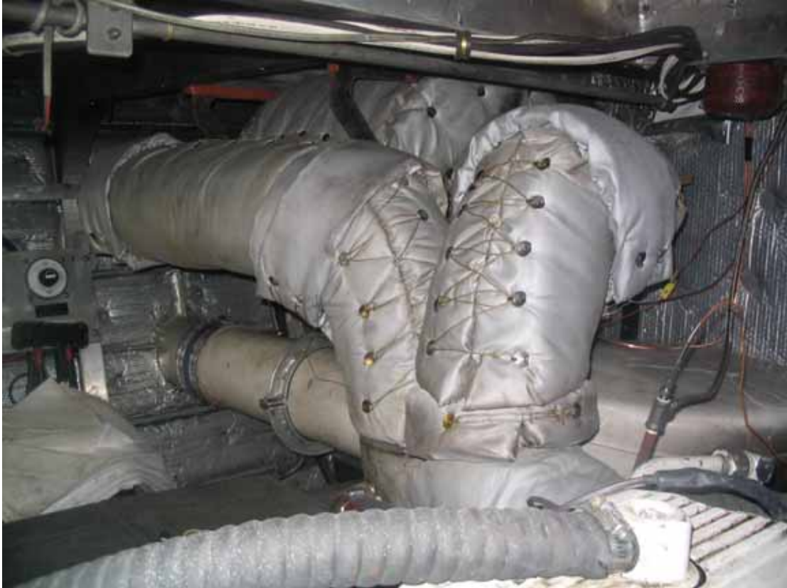
Figure 5.1. MV FATHER MYCHAL JUDGE DOC Installation in Engine Room.
