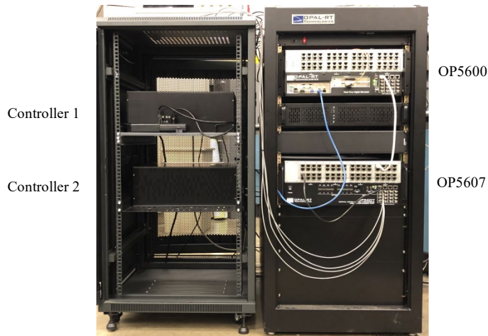
Figure 11. CHIL Setup Overview (Front View)
