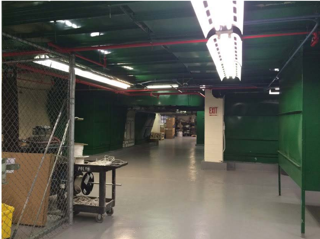
Figure 44. Small parcel of space available in a mechanical room with existing fire suppression system
