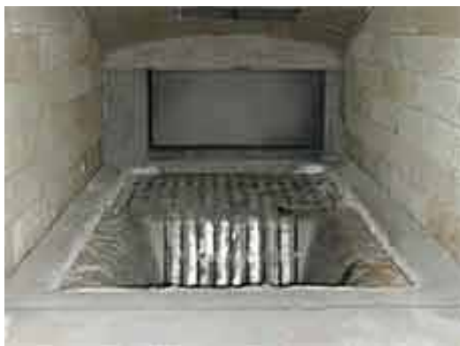
Figure 2-26 Combustion chamber of an underfeed stoker furnace (BINDER 2007)
