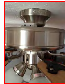
Unable to detect any light from bulbs
