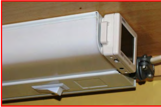
Logger is installed away from the light source and the light sensor is up against the cabinet.
