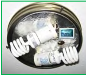
Logger is installed on the base of the fixture; NOTE: Loggers can melt if placed too close to bulbs in an enclosed fixture!
