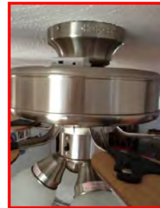
Unable to detect any light from bulbs
