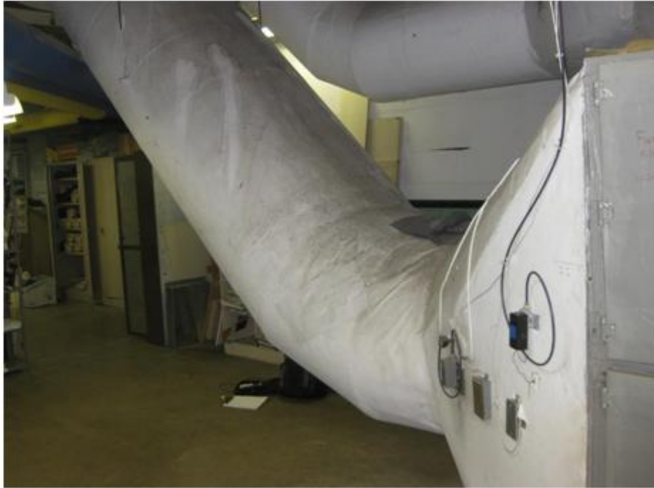
Figure 3-6. Duct System at Project #1, Energy-Efficiency Program Area
