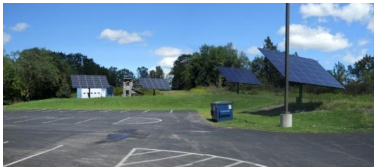
Figure 3-37. Monitored Project Tracking Solar PV System (Multiple Arrays), Renewable Energy Program Area
