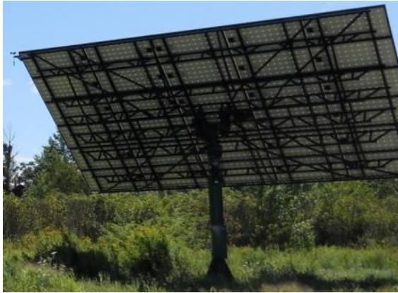
Figure 3-38. Solar Tracker From the Back, Renewable Energy Program Area
