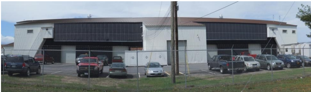
Figure 3-36. Solar Wall Collectors (Exterior View) at Monitored Project, Renewable Energy Program Area
