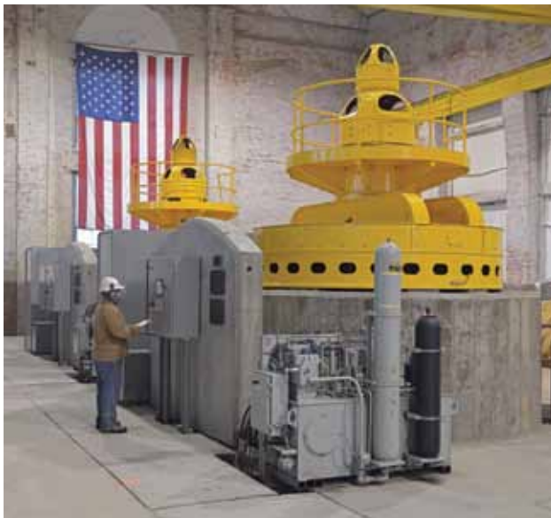
Stuyvesant Falls Hydro
