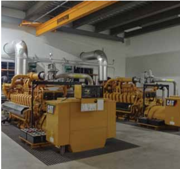
Albany 2 LFG Facility
