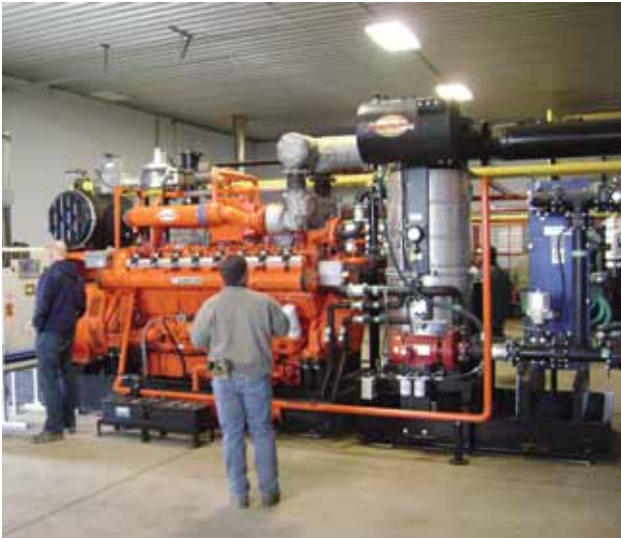
Sunnyside Farms Biogas Engine Generator, Scipio Center, NY
