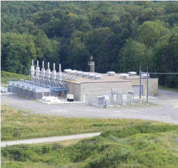
Chautauqua Landfill Gas Facility, Chautauqua County
