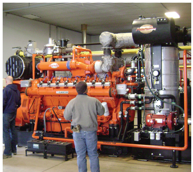
Biogas Generator – NYSERDA photo
