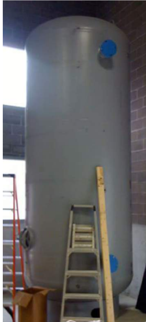
4000 gallon thermal storage tank (before insulation)
