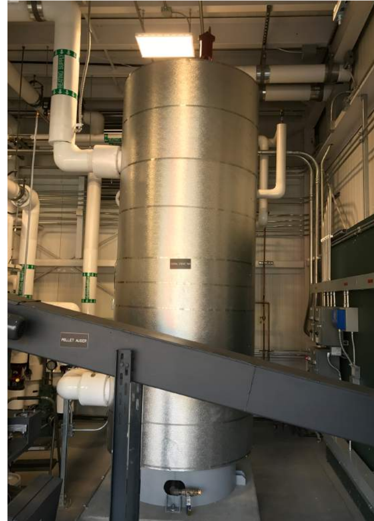
1200 gallon thermal storage tank
