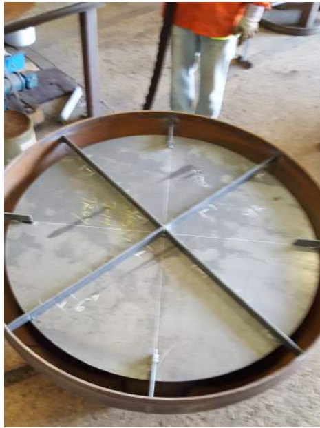
Baffle plate being welded into tank head & base shell at Troy Boiler Works
