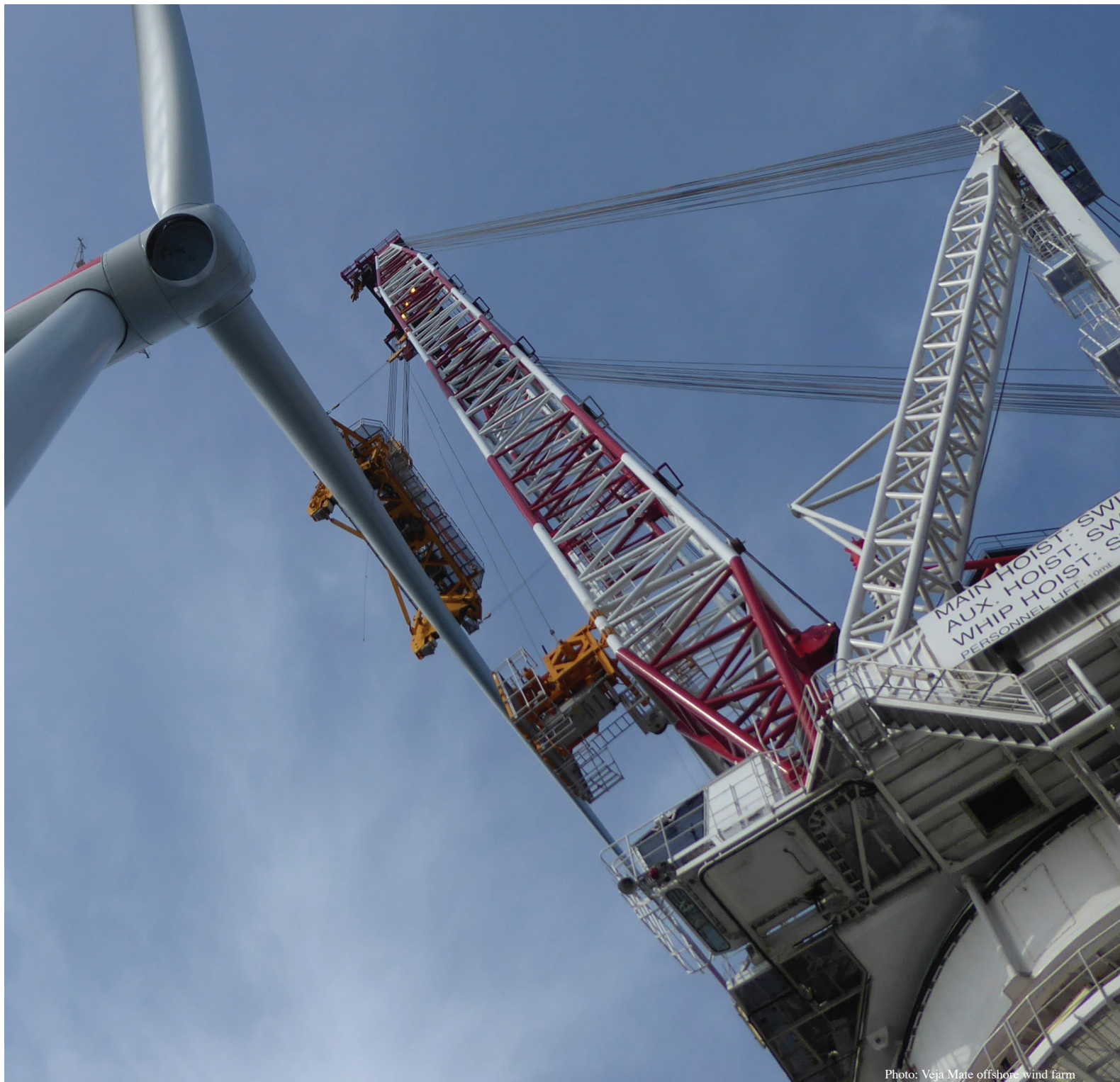
Photo: Veja Mate offshore wind farm
