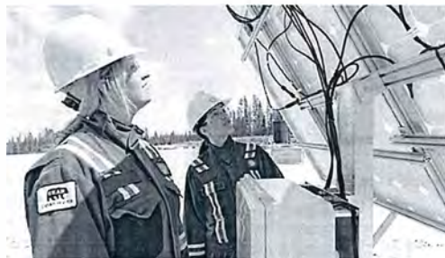
We have installed methane detection technology at our unconventional gas project near Rocky Mountain House, Canada.
