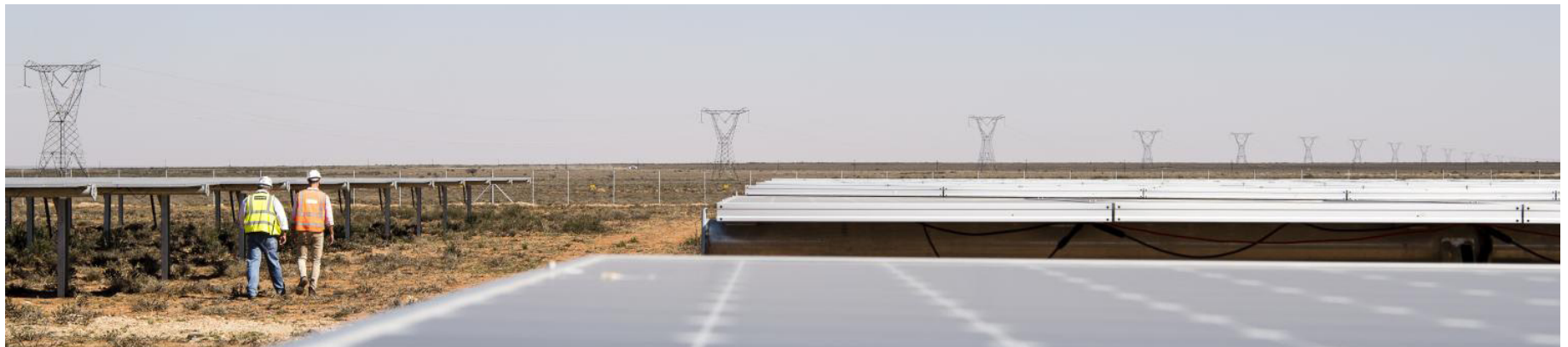
Prieska solar plant in South Africa, which was designed and constructed by TotalEnergies' affiliate SunPower
