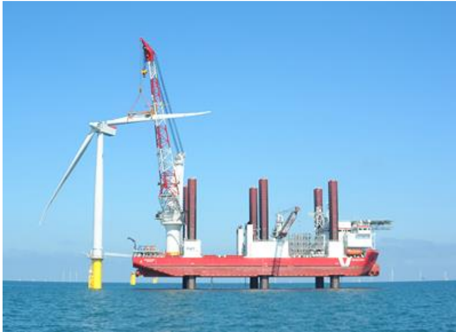
Jack-up barge. London Array Offshore Wind Farm, Thames Estuary, United Kingdom. Photo credit: Siemens Press Picture. 2012.
