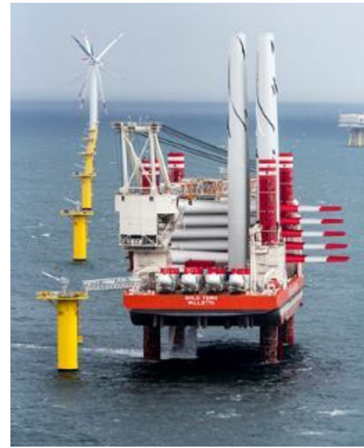
Jack-up barge. Borkum Riffgat Offshore Wind Farm, North Sea, Germany. Photo credit: Siemens Press Picture. 2013.
