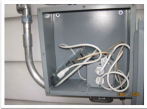
Photo 9: Equipment is not rated for location. In this case, a non-GFCI outlet for PV monitoring equipment is located in a wet location: NEC 110.3(B), 210.8(A)(3)
