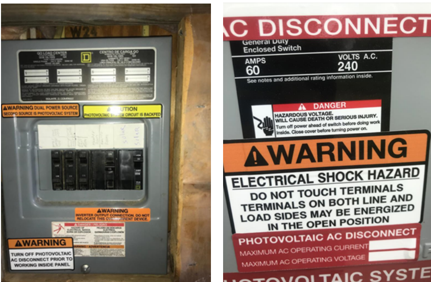
Photo 11: AC disconnect/load center manufacturer's label obscured: NEC 110.21
