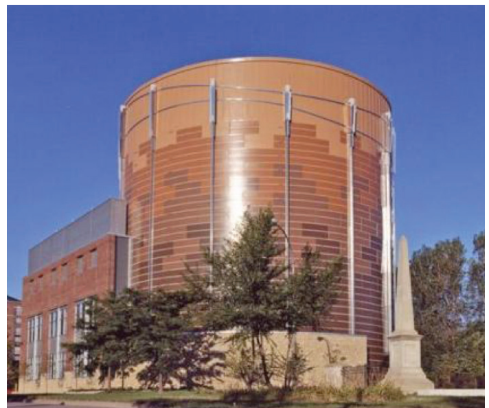
Thermal energy storage tank, District Energy St. Paul. Photo by Ever-Green Energy.
