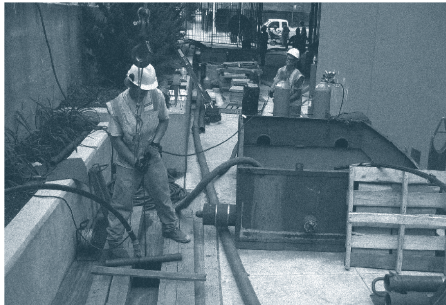
Technician lowering tool into well
