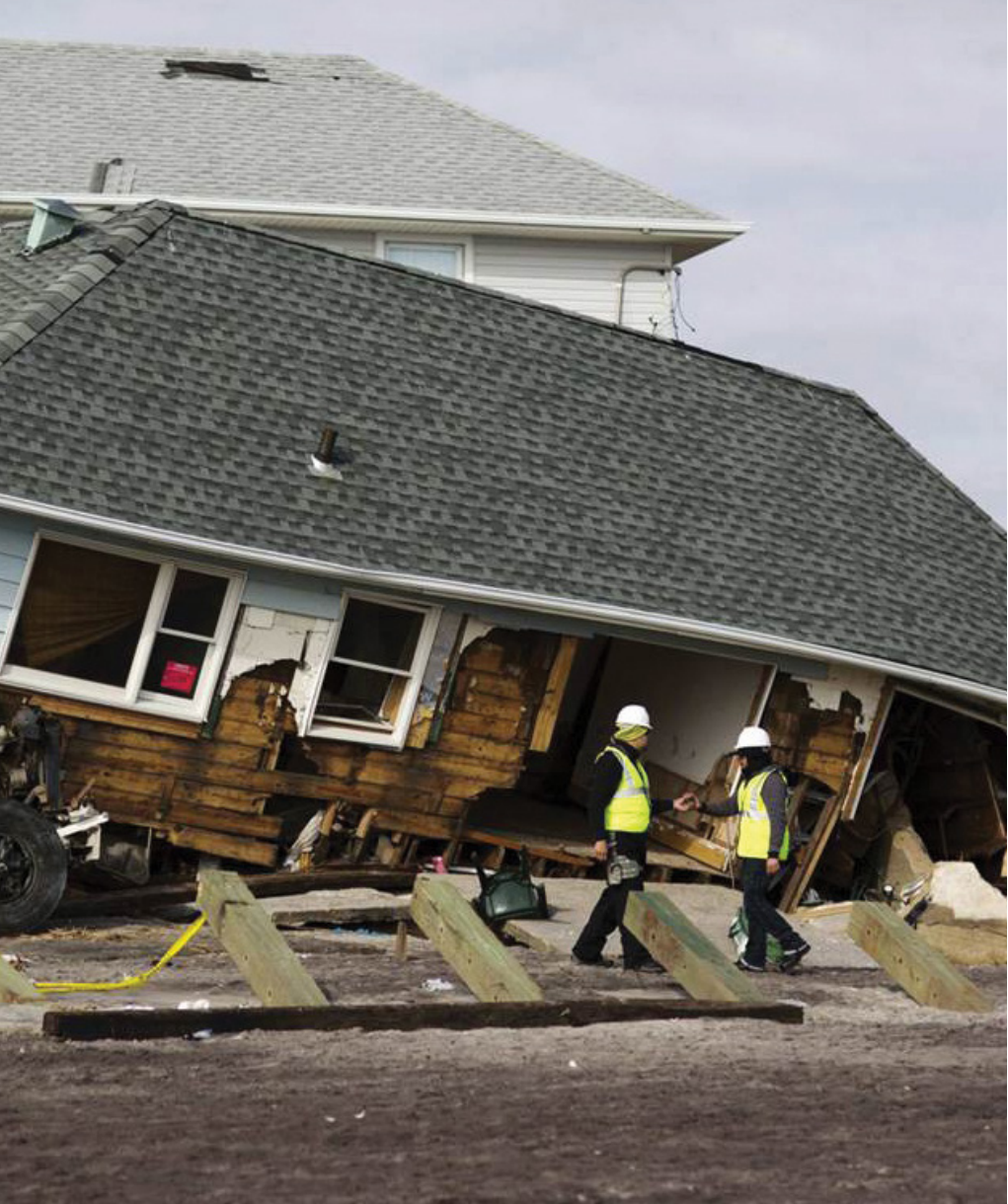
Home destroyed in Belle Harbor. Photo Source: New York State Division of Homeland Security and Emergency Services
