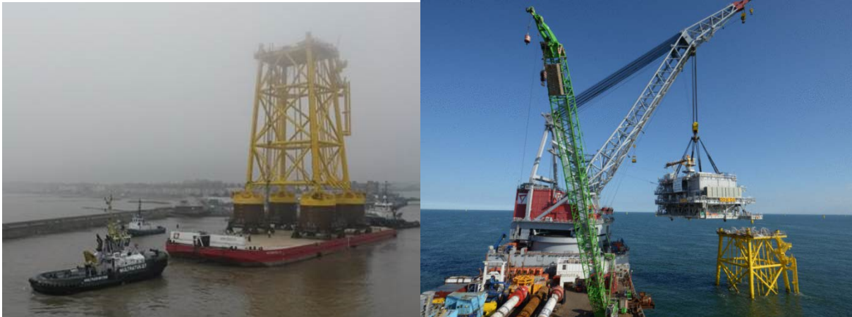
Figure 88: Dudgeon Offshore Substation Jacket on Barge (Left) Typical HLV Used for Offshore Substation Installation (Right)
