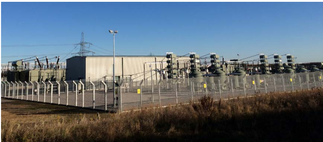
Figure 58: Dudgeon Onshore Substation
