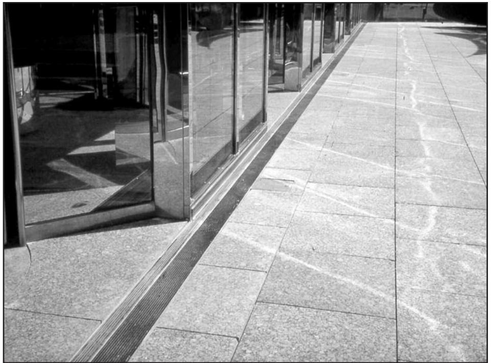
Figure 15 – Gutter drain at access door with ADA grating.
