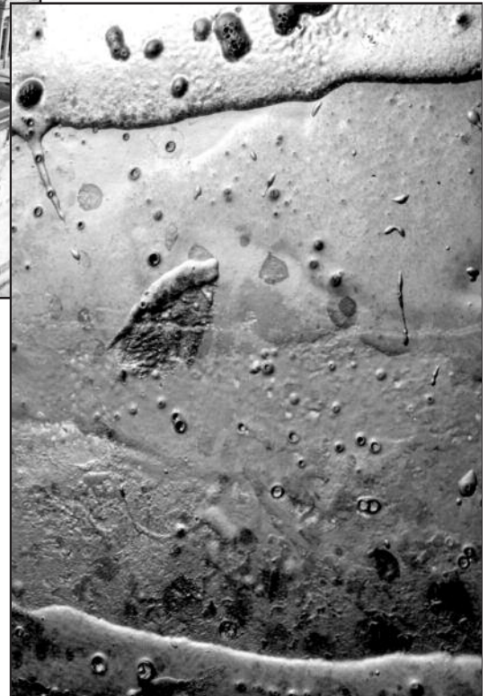
Figure 7 – Pinholing and air bubbles in liquid-applied membrane.
