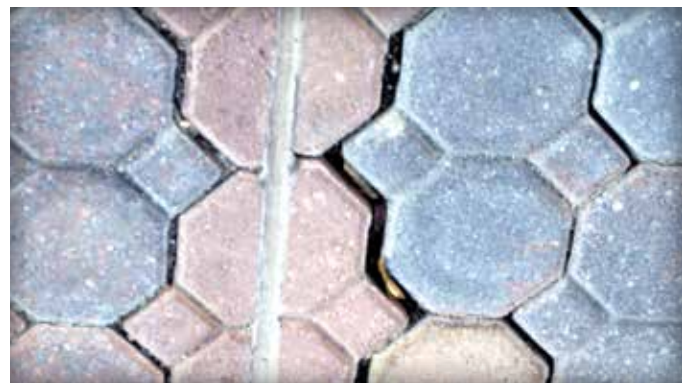
Figure 13. An absence of edge restraints and use of a sealant in this construction joint caused the pavers to shift and open their joints on both sides of the sealant.
