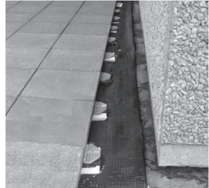
▲ Installation of a paver-on-pedestal system. Pavers are supported only at corners, with fully open joints.
