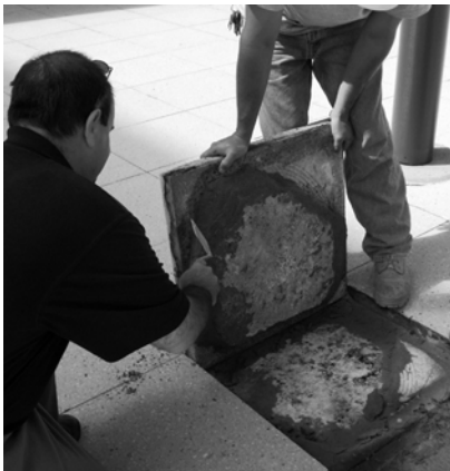
▲ Plaza investigation by an experienced architect or engineer uncovers the causes of water damage or deterioration.
