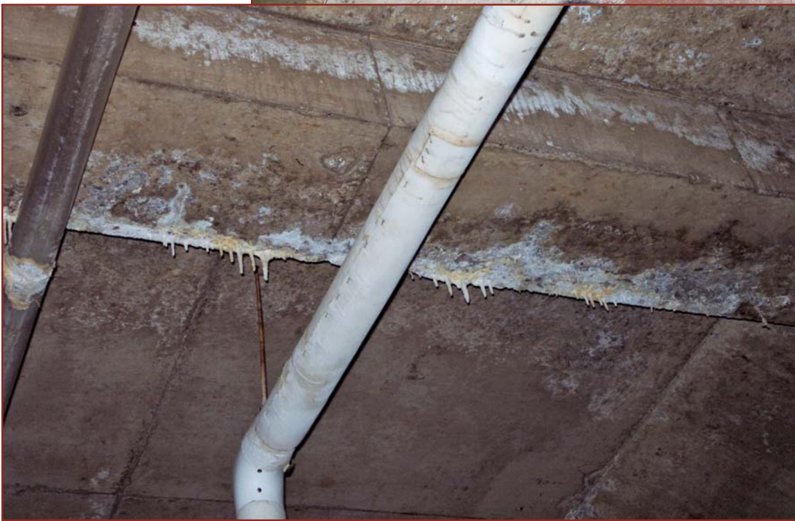
Photo 5 – Leakage to interior spaces below a plaza.
