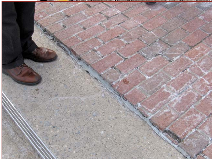
Photo 3 – Frost heaving of brick pavers.
