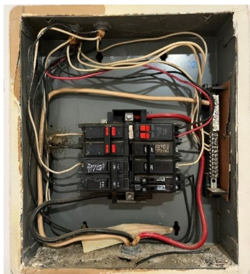
Figure 6. Site 2 Electrical Panel
