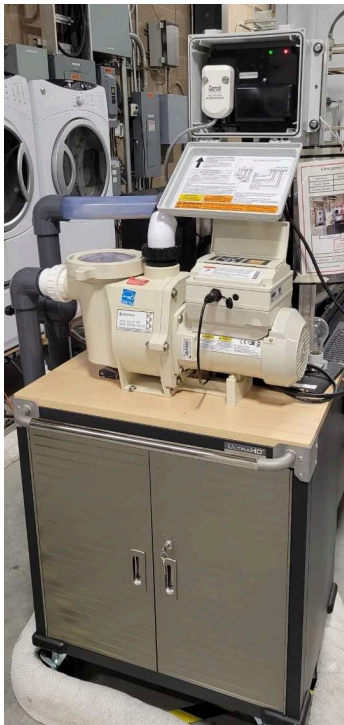
Figure 22. Lab Test Setup for Pool Pump Controller
