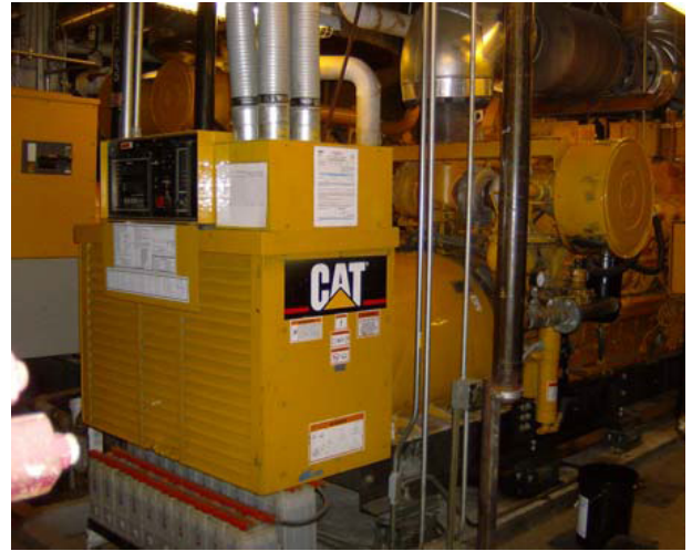
Caterpillar Engine Generator
