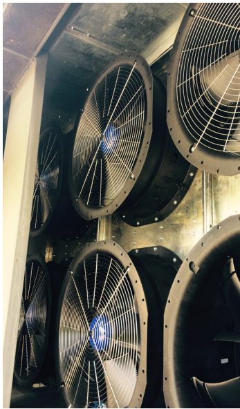
One cell fan wall cooling tower
