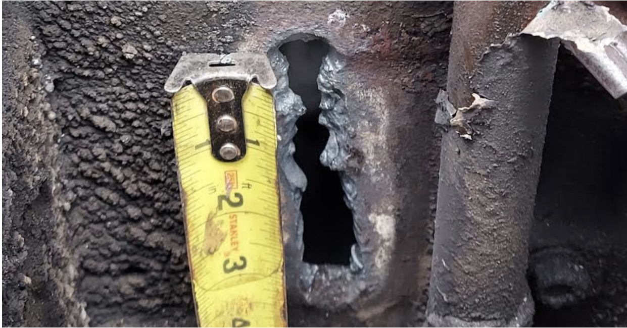
Figure 12. In a case where NYSERDA stickers are not available, a tape measure can be used to document the appropriateness of the size of the hole drilled in an engine block.
