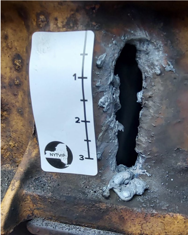
Figure 8. An “after” photo of a drilled engine block with the accompanying NYSDERDA sticker for documentation.
