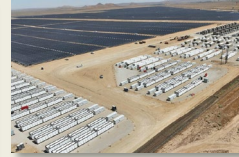
Energy Storage BESS
