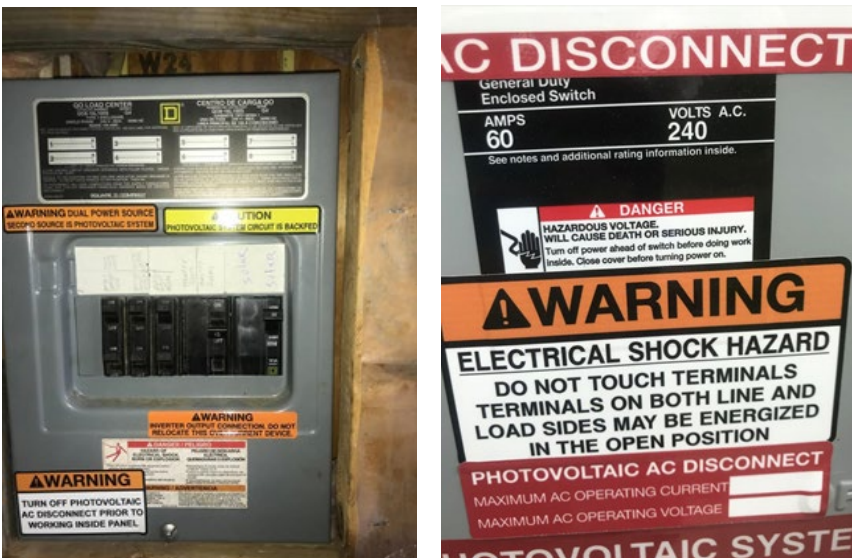
Photo 11: AC disconnect/load center manufacturer's label obscured: NEC 110.21
