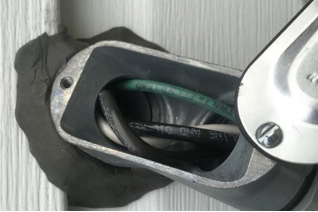
Photo 13: Two Hole conduit strap, with only one point of attachment, and no strain relief on conductors: NEC 110.3(B)
