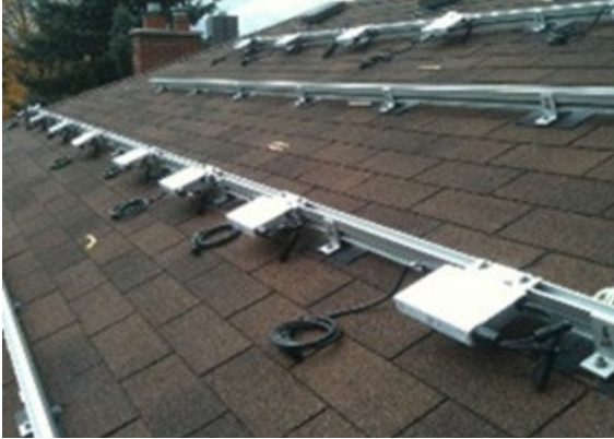
A Solar Electric Racking System
