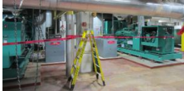
MV Generators at RCPI (3rd Floor Plant Electrical Room)
