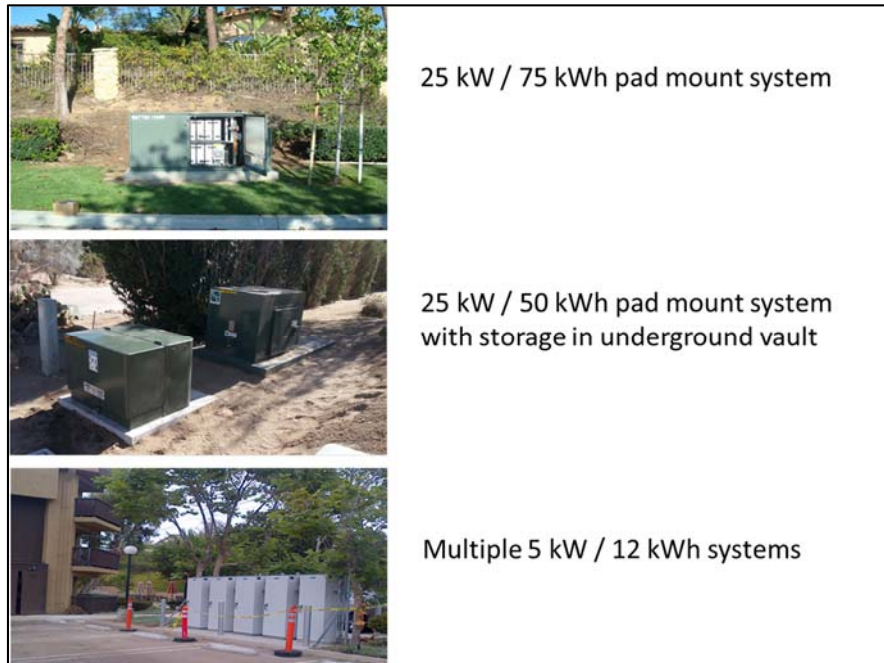
Figure 2.12 – Example ESS Installations
