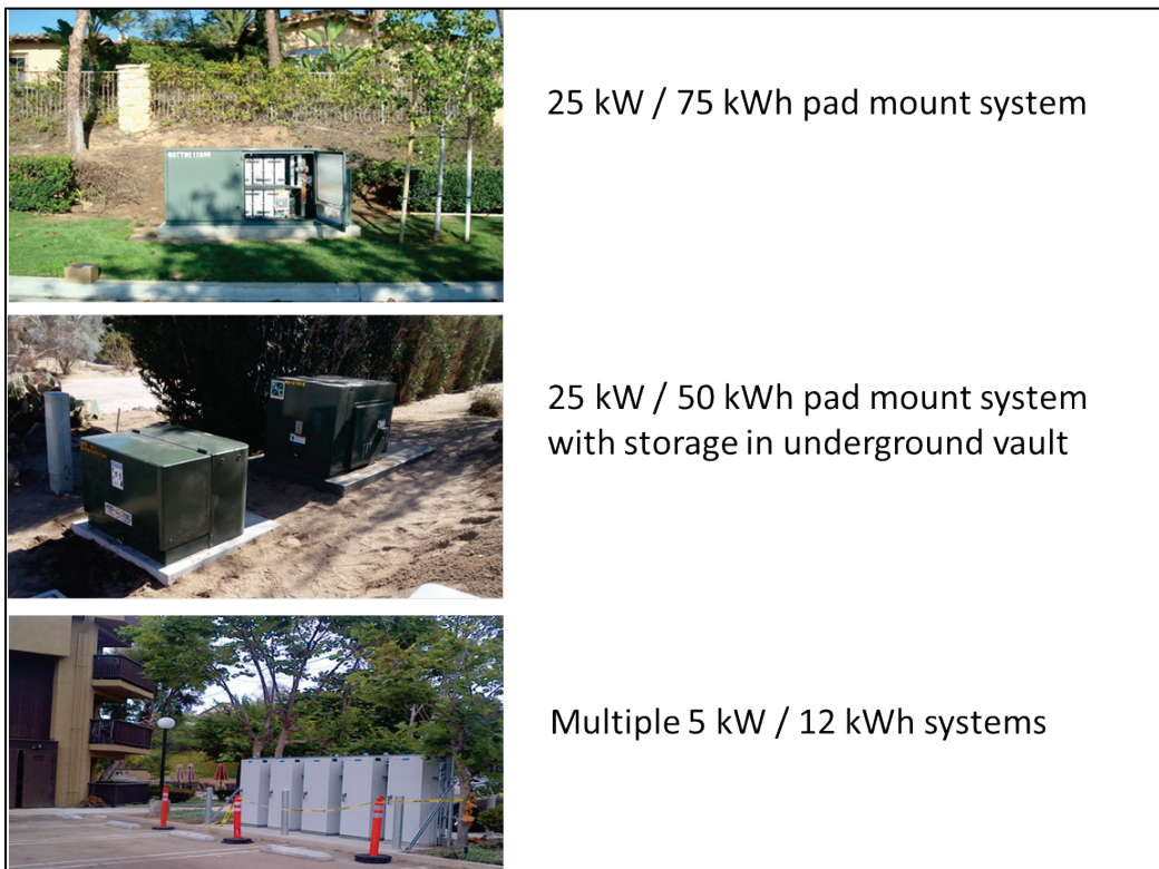
Figure 16 – Example ESS Installations
