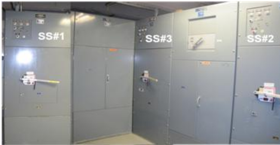
Photo 2-4. Brookhaven Town Hall Service Switchboards
