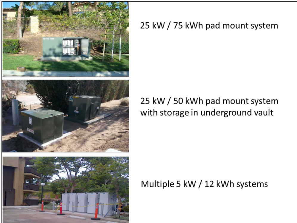
Figure 17 – Example ESS Installations
