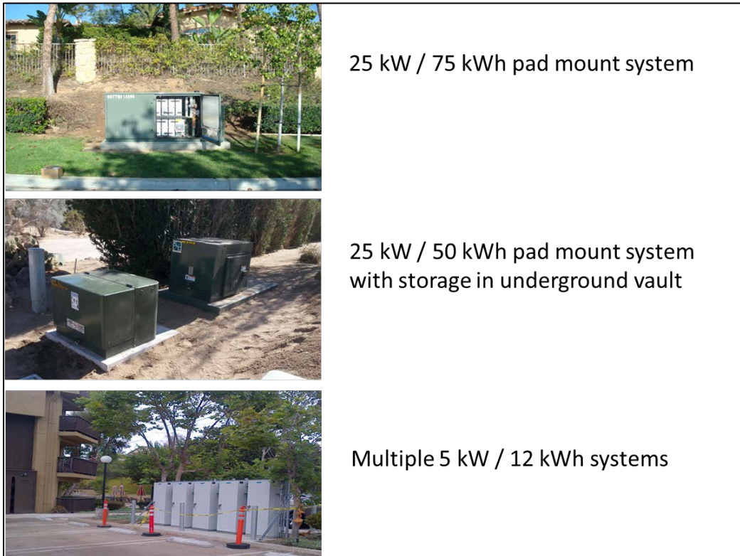
Figure 16 – Example ESS Installations
