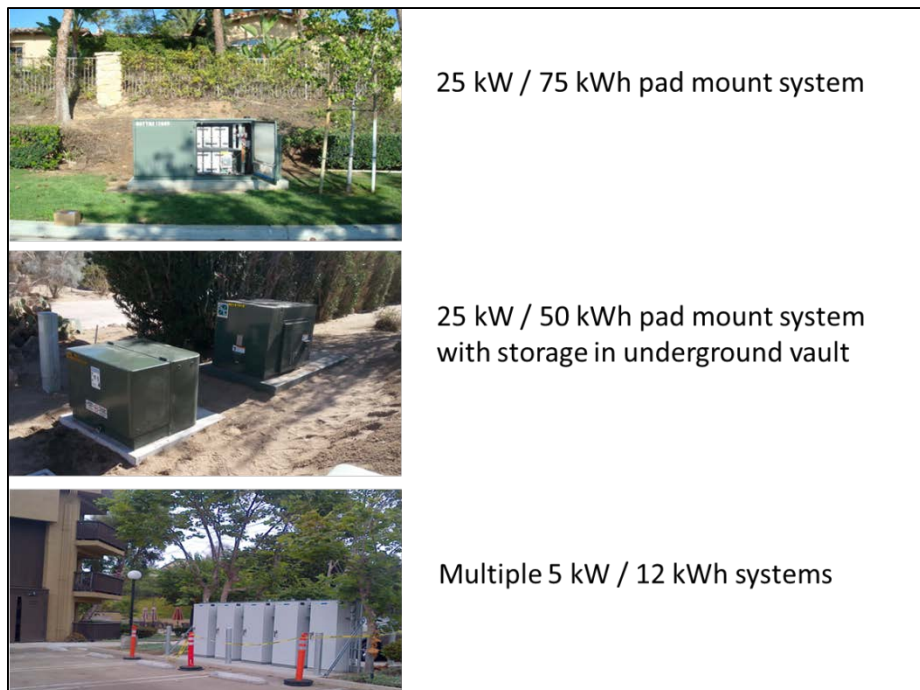
Figure 11 – Example ESS Installations
