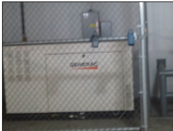
Figure 36. Backup Generator: The Regatta
