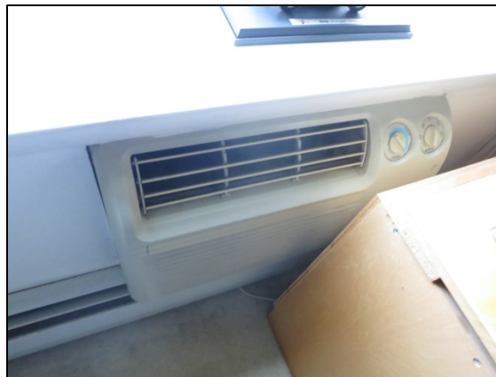
Figure 34. Typical living room PTAC: The Regatta
