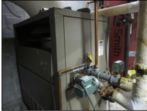
Figure 35. DHW Boiler: The Regatta
