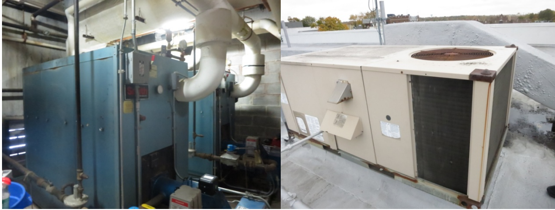
Figure 33. Gas Fired Boilers (left) and Gas-fired RTU (right): The Regatta
