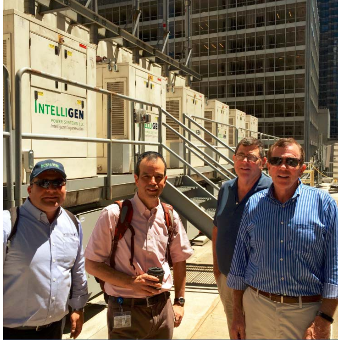
Figure 56. Sean and Chris Murphy join VOM Microgrid team member Sal Cona, from Intelligen, and Mick Gilbert from Con Edison for a tour of a large Co-Gen installation in midtown Manhattan
