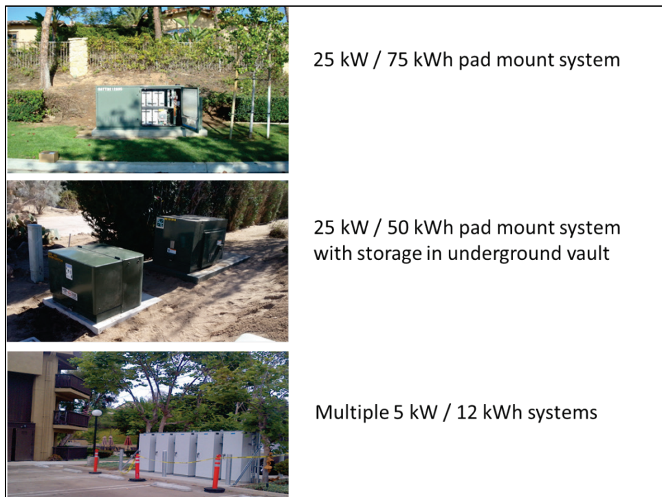
Figure 16 – Example ESS Installations
