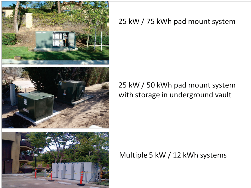
Figure 16 – Example ESS Installations
