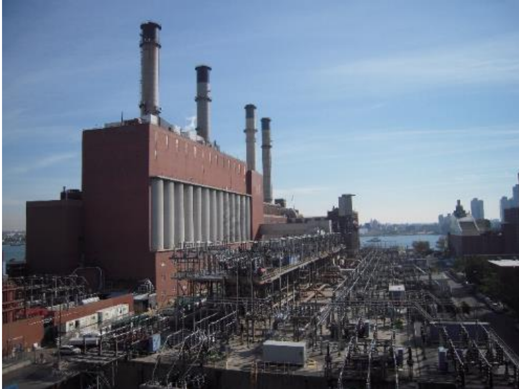
Figure T3-9 Across Ave C from Campos Plaza is a ConEd substation that was disabled by Sandy; the microgrid (especially as it grows) will be able to assist in the substation's resiliency.
