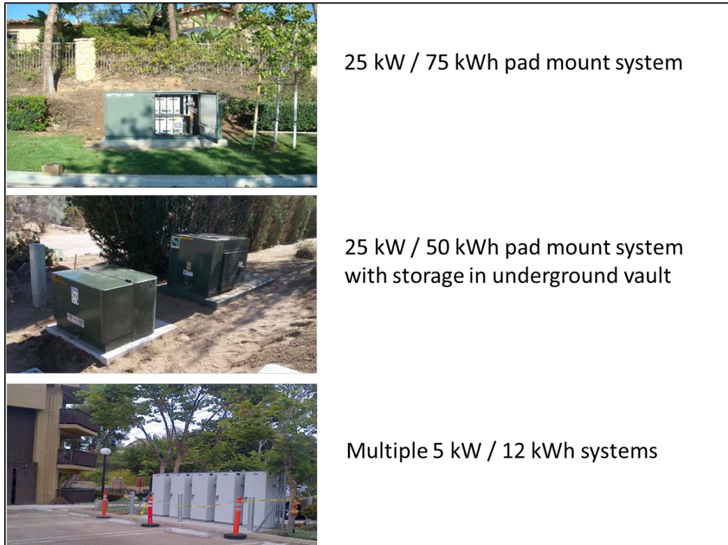
Figure 16 – Example ESS Installations
