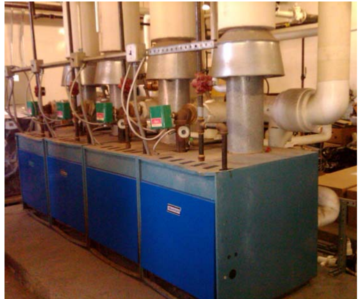
Fig. 2 Cast Iron Sectional Boilers
