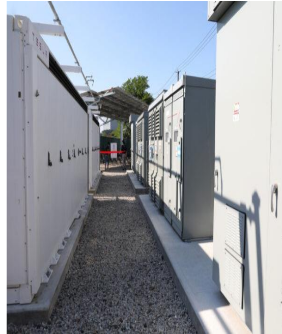
Off-Site Retail “Front of the Meter” ~1-5 MW
