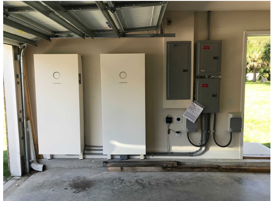
9.8 kW / 20 kWh installation: SonnenCore+ , (4.8 kW / 10 kWh/unit); installed in garage
