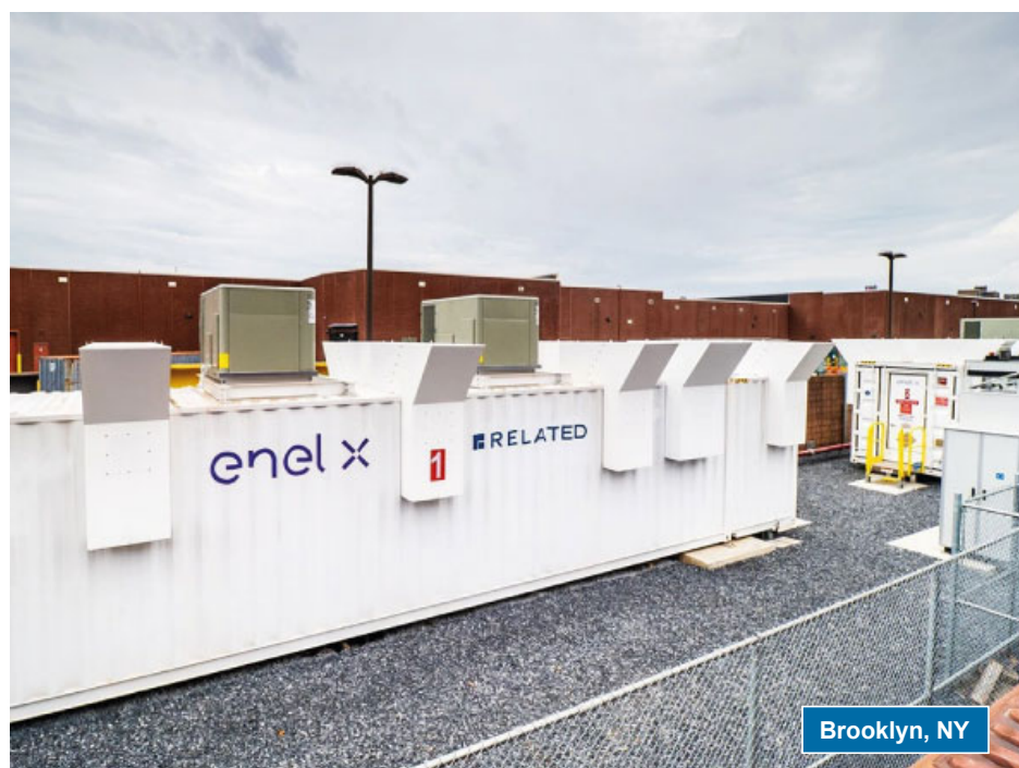
4.8 MW / 16.4 MWh installation: Enel X's Gateway Center project ; sited at a commercial shopping center in Brooklyn, NY
