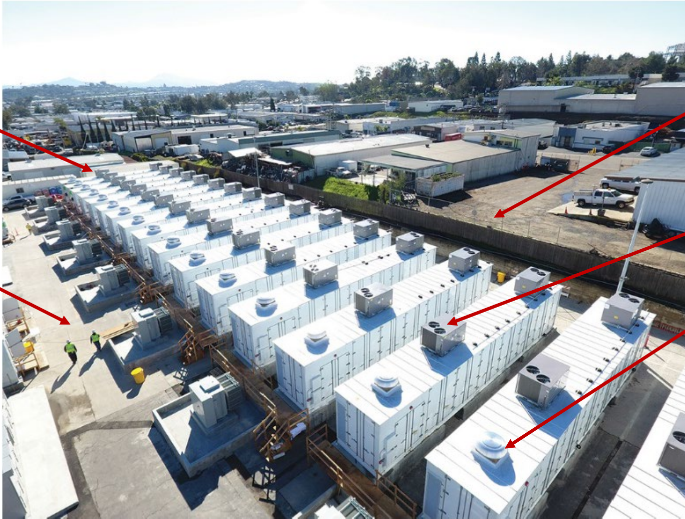
SDGE, Escondido 120 MW installation
