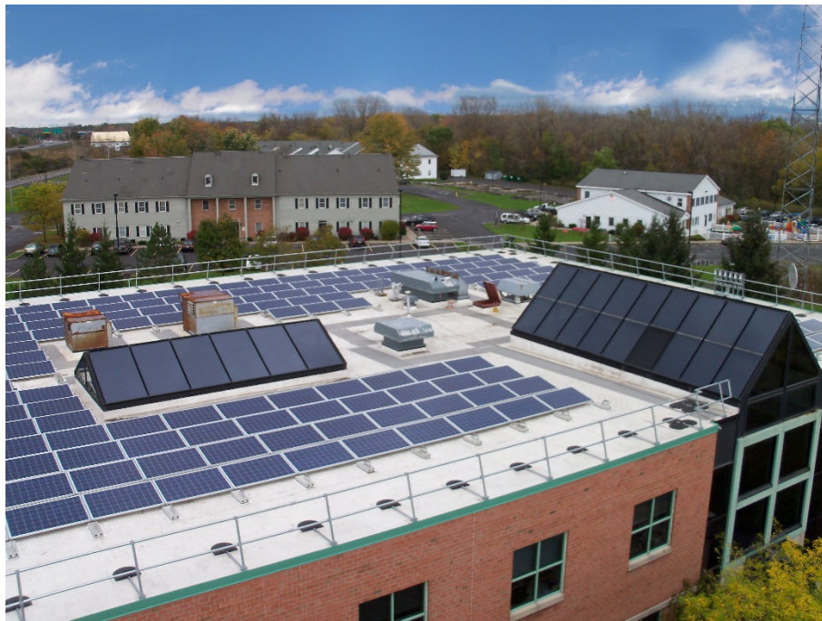
51 kW PV Array – Town of Dewitt, NY
