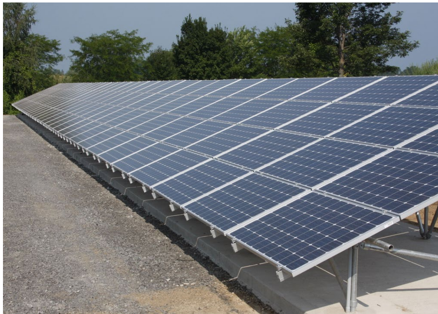
Town of Williamson, NY Solar Array
