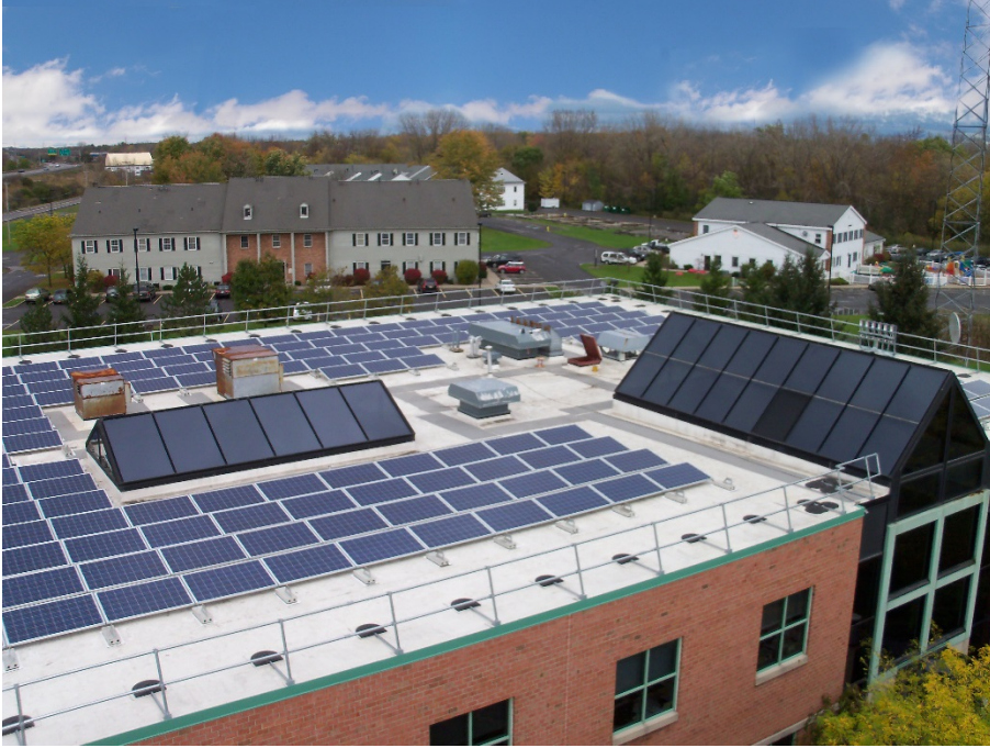
51 kW PV Array – Town of Dewitt, NY
