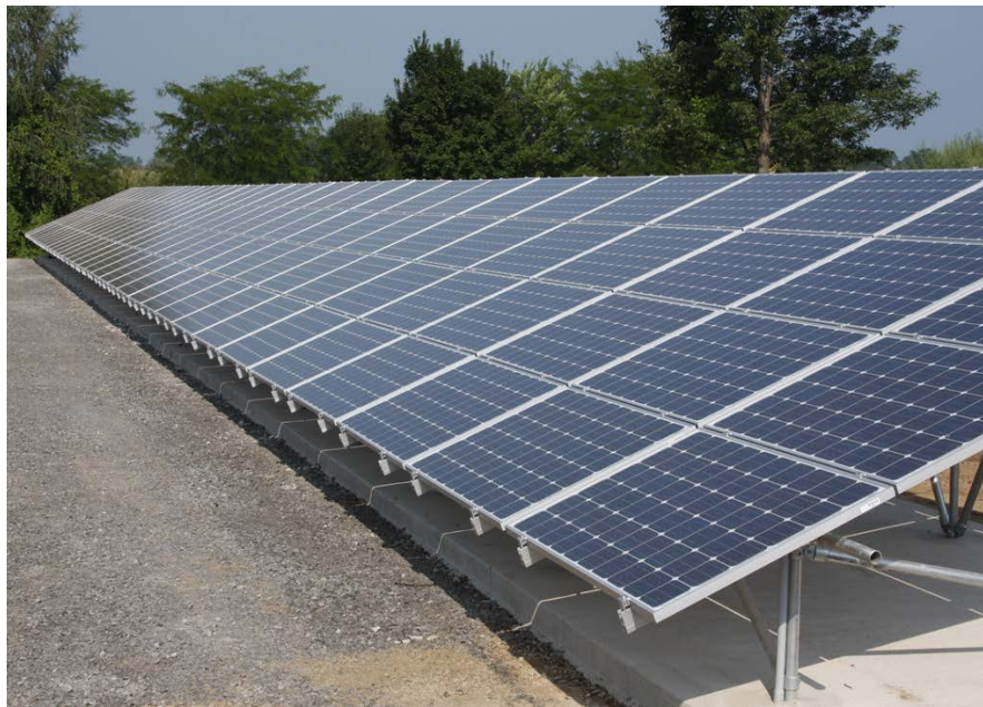
Town of Williamson, NY Solar Array
