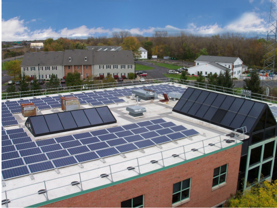
51 kW PV Array – Town of Dewitt, NY
