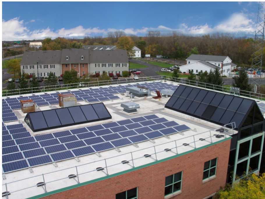
51 kW PV Array – Town of Dewitt, NY
