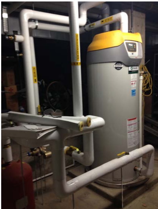
New Domestic Hot Water System City of Lockport, NY
