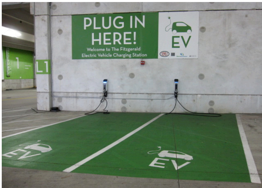
Figure 2. Charging stations at the Fitzgerald
