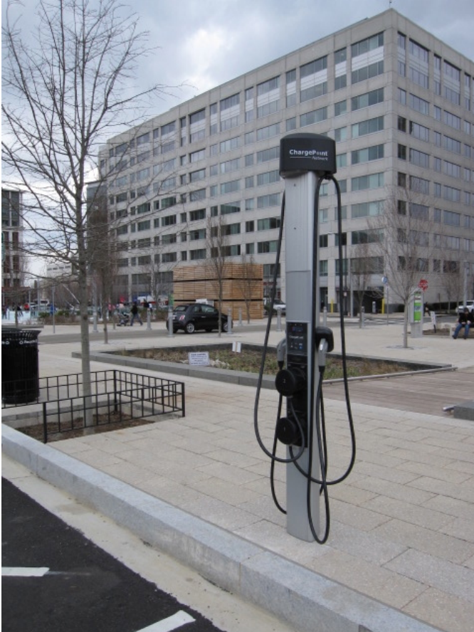
Figure 14. Dual level 2 charging station at Canal Park
