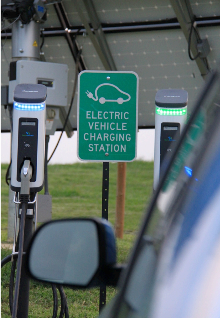
Figure 13. Charging station and solar tracker at Linganore
