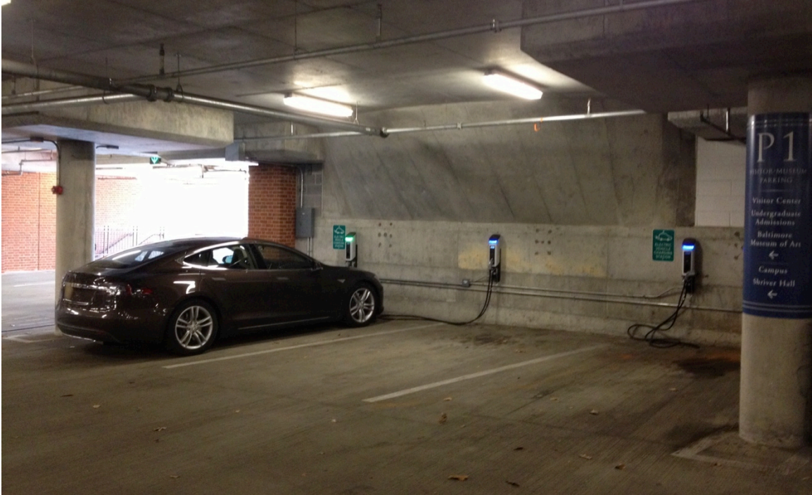
Figure 28. Charging stations next to garage entrance
