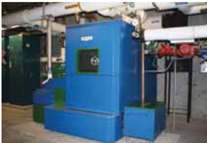
ACT Bioenergy equipment at The Wild Center in Tupper Lake, New York.
